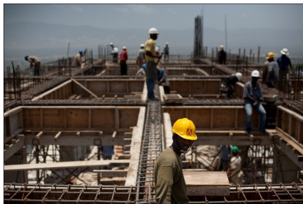
Top to bottom: The hotel approaches its final stages; Ongoing construction of the hotel.
