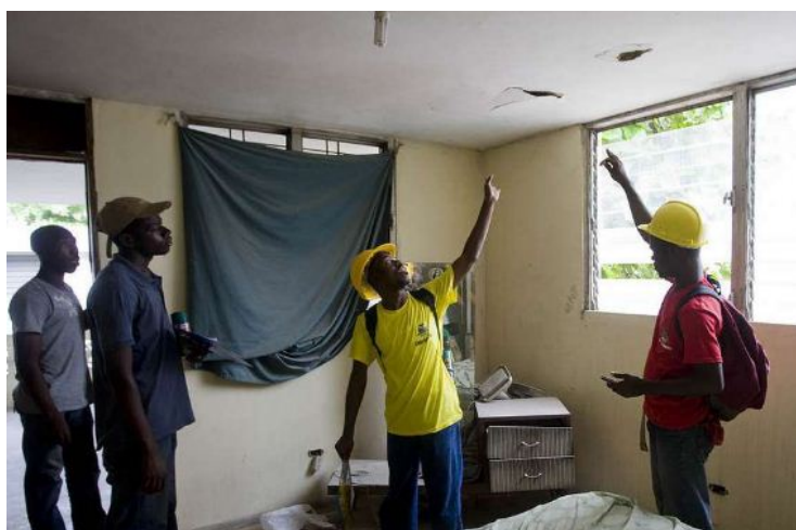
Trained contractors assess the damage in a yellow tagged house.
